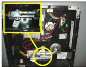
Water heater drain plug
